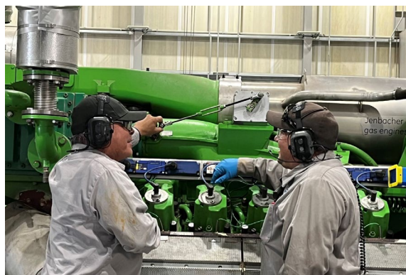
Mechanics working on the cogeneration engine
