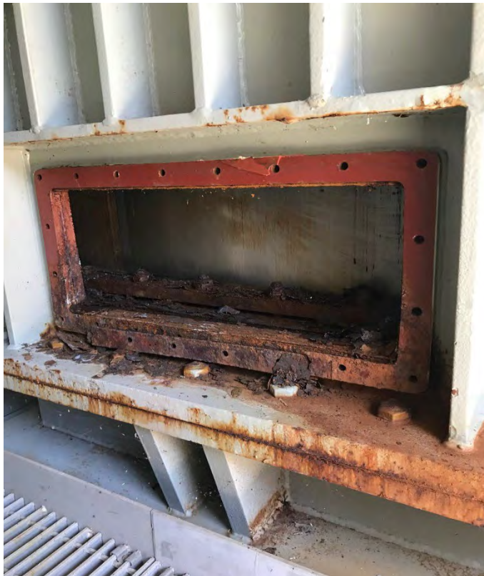
Figure 4 –Corrosion at Maintenance Access on Upper Section of the West Knife Gate Valve at Headworks Valve Box
