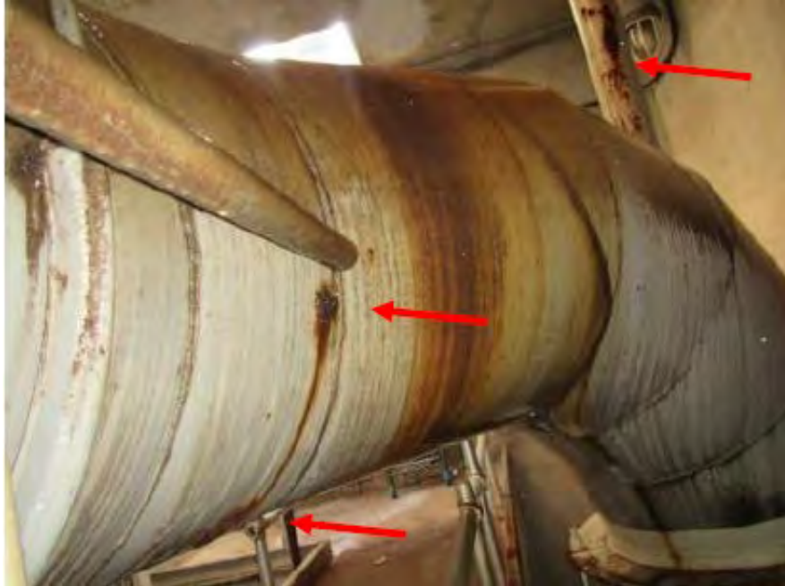
Figure 5 – Exterior corrosion on pipe at the Alvarado Influent Valve Box
