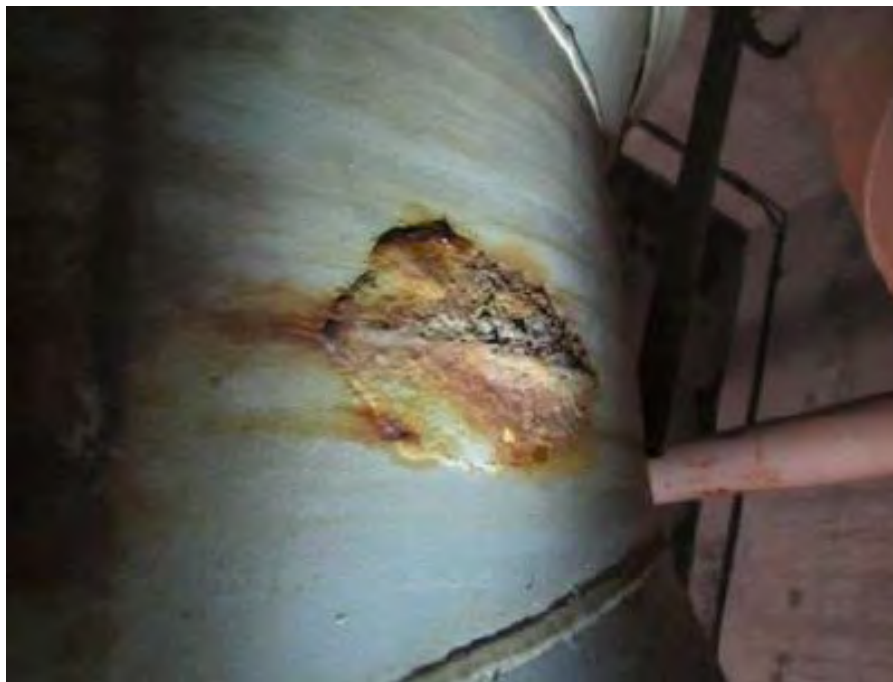
Figure 6 – Detailed view of corrosion at on pipe at the Alvarado Influent Valve Box
