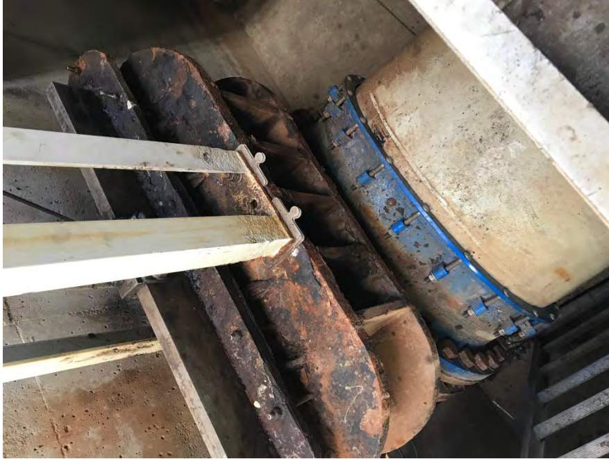
Figure 3 – East Knife Gate Valve at Alvarado Influent Valve Box
