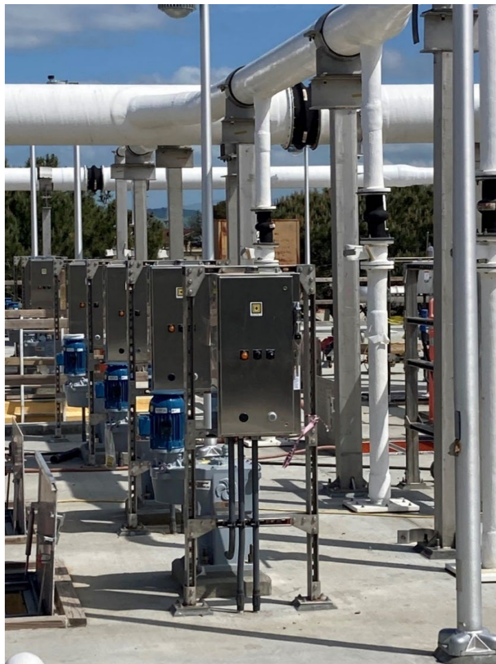
Motor Control Panels at New Aeration Basins
