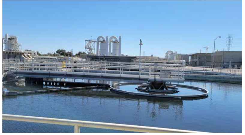
Clarifier- Treatment Plant
