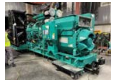
Standby Power Generator
