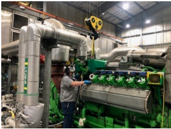
Preventative Maintenance: Cogen
