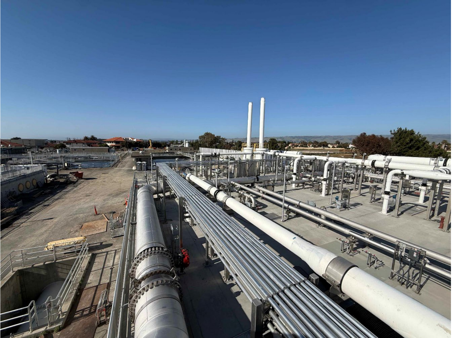
Refurbished Easterly Aeration Basins – Air Supply, Duct Bank and Foul Air Return
